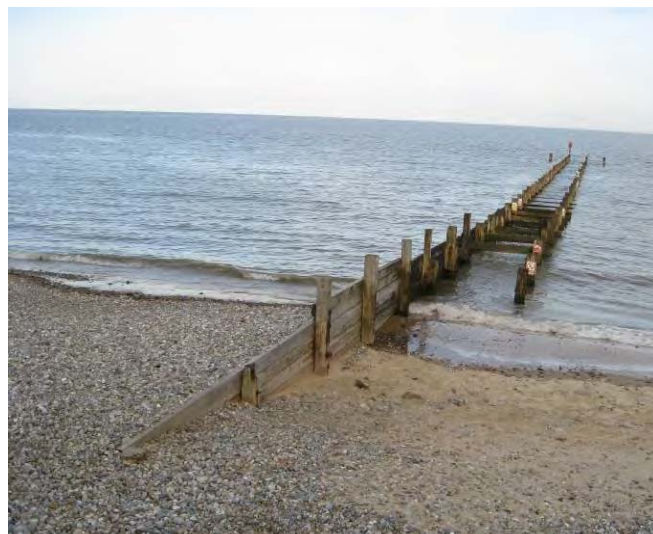
Figure 2-14 Pile-group Kingpile timber groynes at Lowestoft. A dual row of king piles is used to create an access platform for piling plant, allowing construction of groynes below the low water mark. Photograph taken 21/05/09
