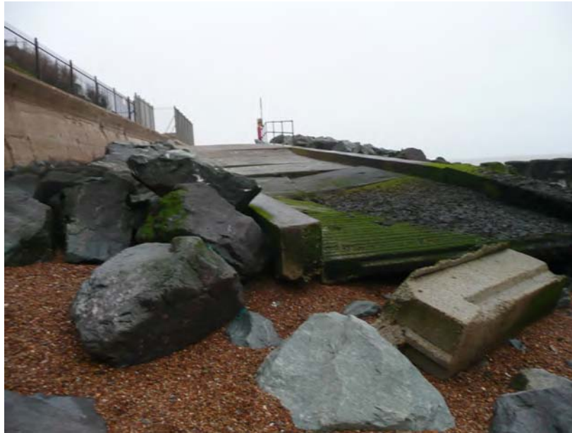
Figure 2-5 Collapsed access slipway at Cobbold's Point.
