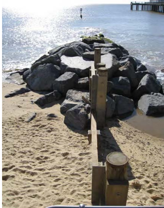
Figure 2-15 One of the 2005 rock groynes at Southwold. The rock groynes were carefully constructed to reduce the voids between the rocks in an attempt to reduce health and safety issues. The head of the groyne at the seawall has removable timber struts to enable access. Photograph taken 22/05/09
