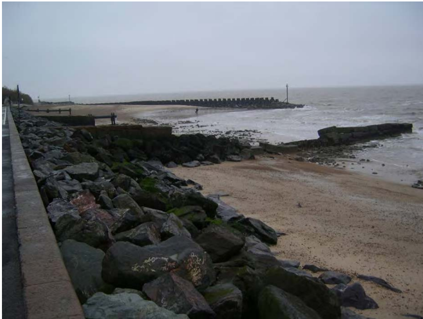
Figure 1-2 Collapsed concrete encased timber groyne and lowered beach levels outside the Fludyer's Arms (February 2009).
