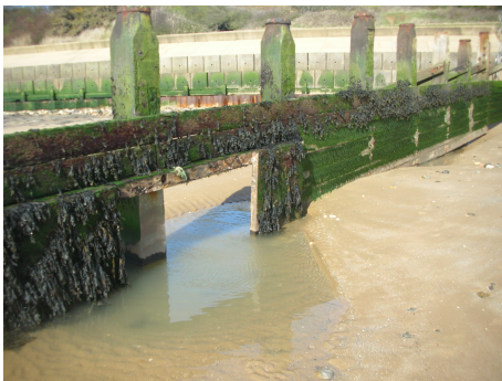
Figure 17: Missing Boards Cause Erosion a
