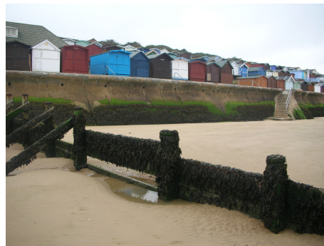
Figure 18: Missing Boards Cause Erosion b
