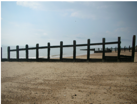
Figure 11: Holland Top Plank Bolted
