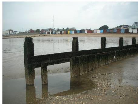
Figure 20: Missing Boards Cause Erosion d
