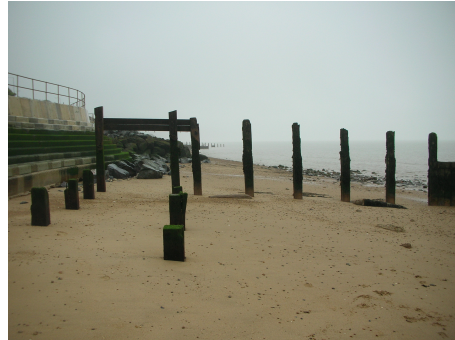
Figure 16: Missing Boards Cause Erosion d
