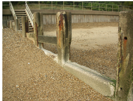
Figure 12: Holland Groynes Fill a
