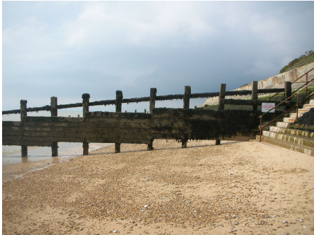
Figure 15: Missing Boards Cause Erosion c
