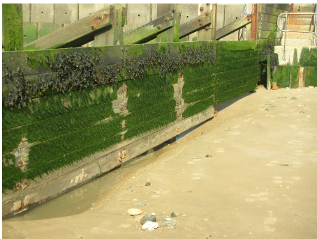
Figure 19: Missing Boards Cause Erosion c
